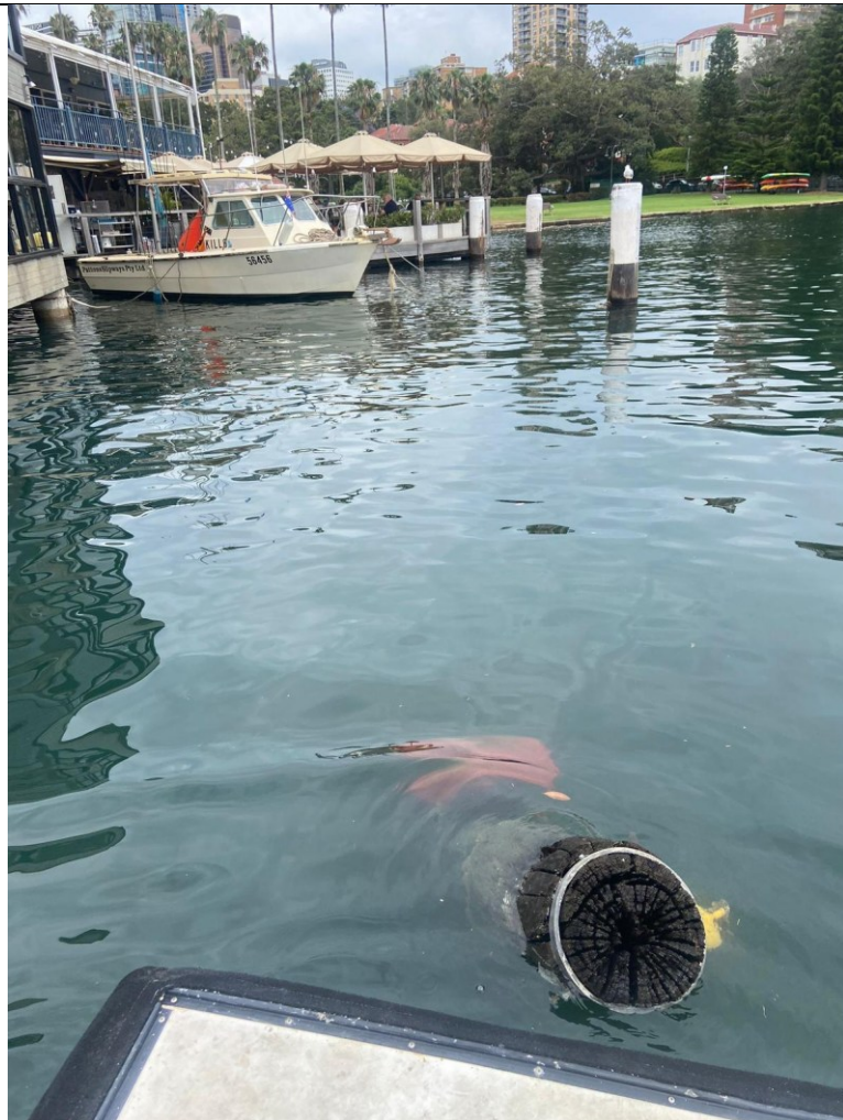
The collapsed mooring pile from last week
